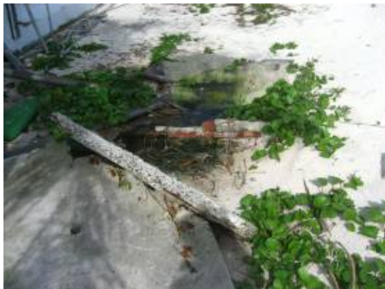
(A)化糞池破損外漏
